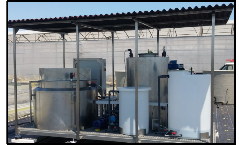
Pilot plant 1 m 3
