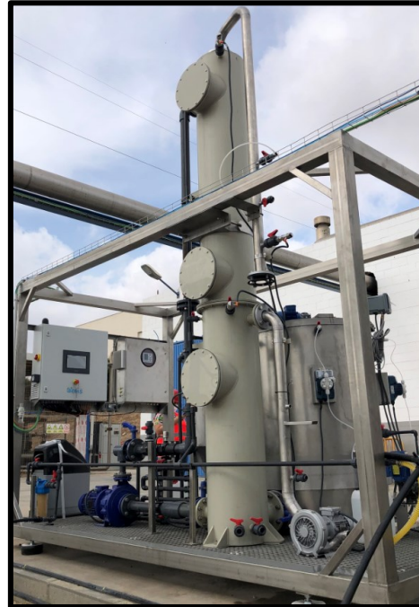
Pilot plant 1 m 3
