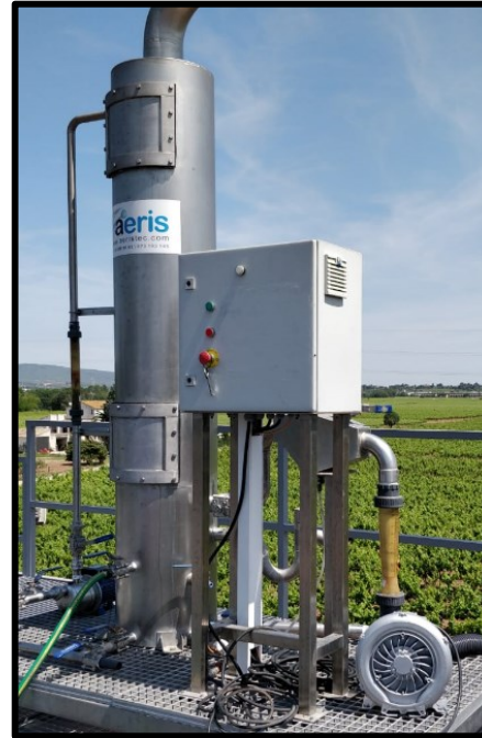
Pilot plant 150 L
